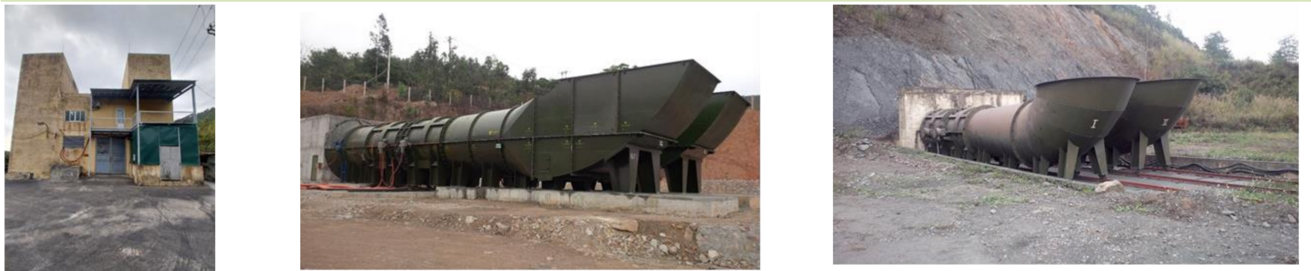
Fig.2. Image of main fan station 2K56-No24 at the door of tunnel the level +69, level +120, level +45
